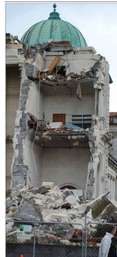
Catholic Cathedral damaged in Christchurch earthquakes
